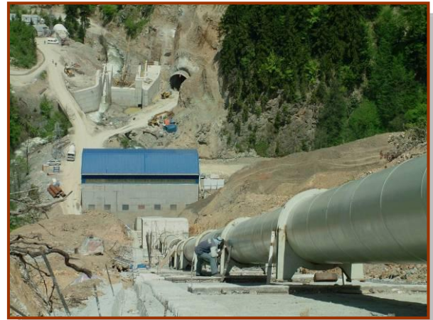
This photo shows how the tail water of a HEPP is immediately taken in by the next HEPP. Photo Source: Dr. Oğuz Kurdoğlu
